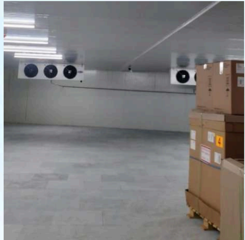
Multipurpose Cold Storage
