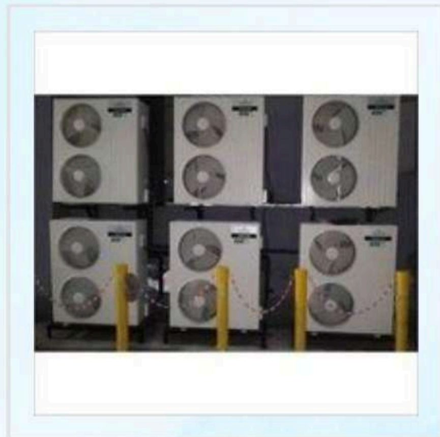
Cold Room Outdoor Unit
