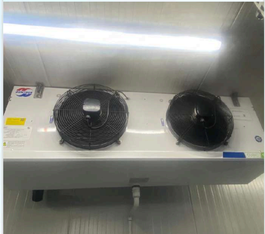
Evaporator unit cold storage
