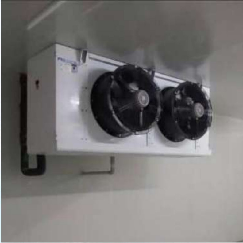
Automatic Cold Storage Room
