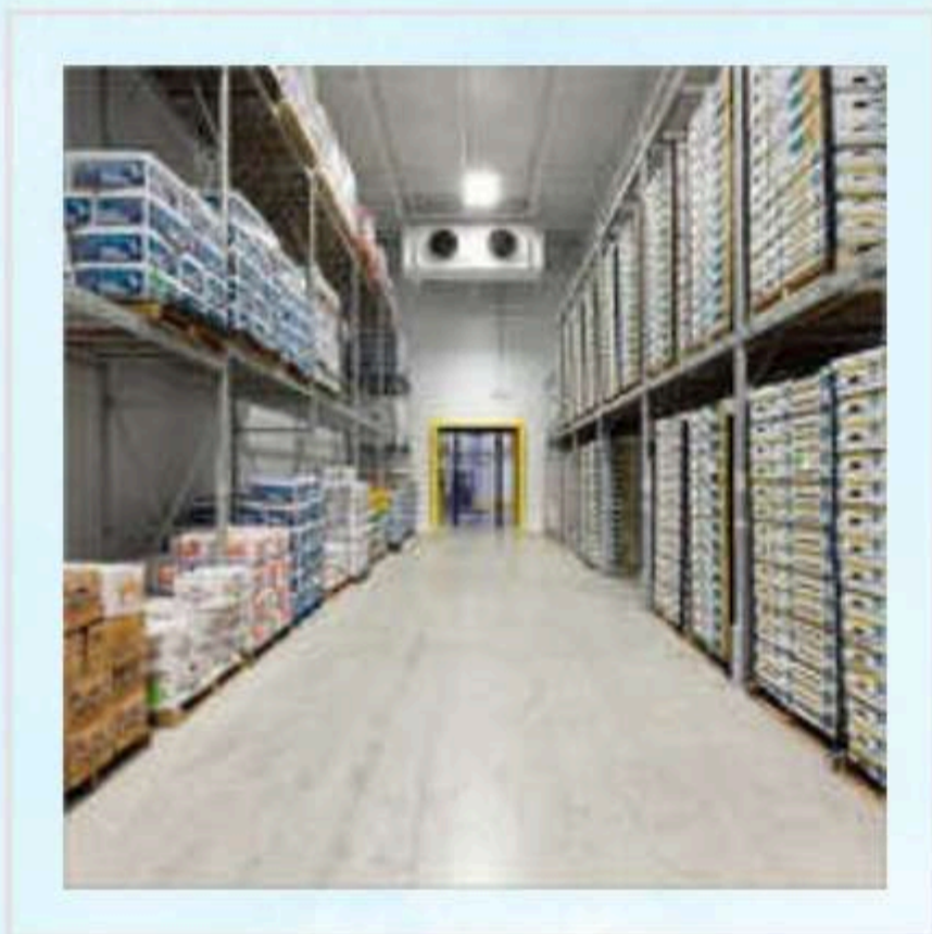
Industrial Cold Storage Room
